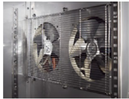
蒸發器 Evaporator compartment
